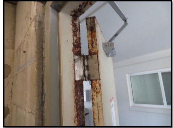
Figure 2 – Corroded Door Frame
