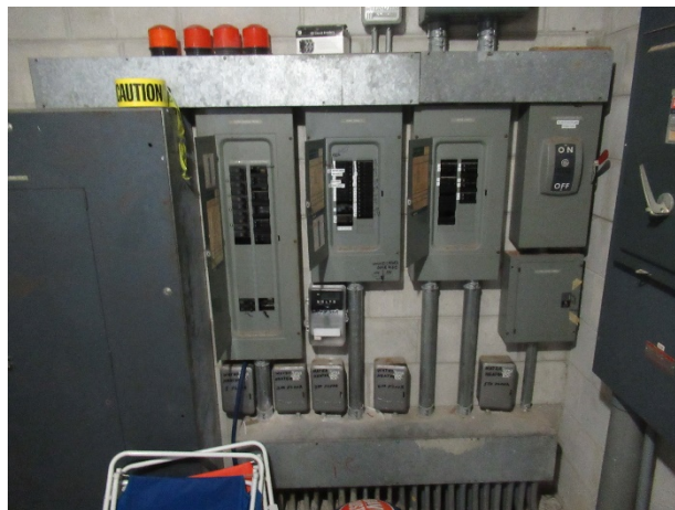
Electrical system components
