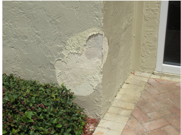
Stucco not yet repaired
