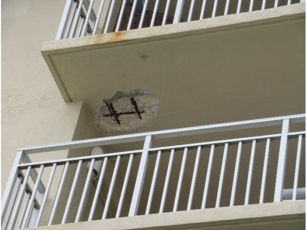
Balcony with significant spall and exposed reinforcing steel
