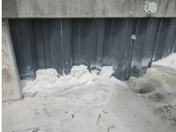
Vinyl bulkhead with wash-out near drain
