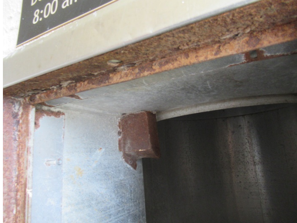
Rust at door and collar to be replaced
