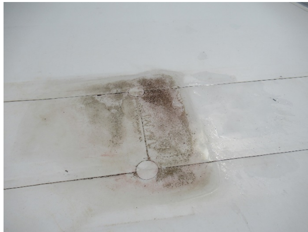
Stains and ponding water
