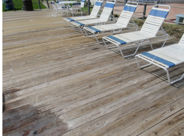
Weathered deck boards
