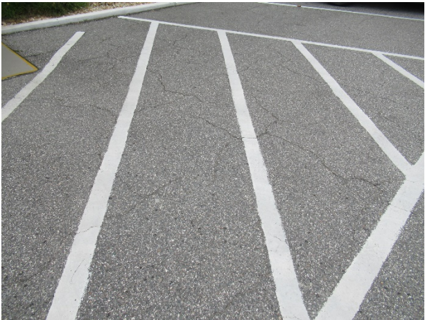
Asphalt pavement with block cracks
