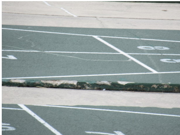
Deterioration to shuffleboard courts
