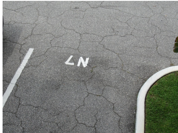
Asphalt pavement with block cracks
