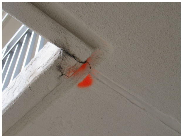
Crack to breezeway underside to be repaired
