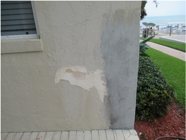
Stucco not yet repaired
