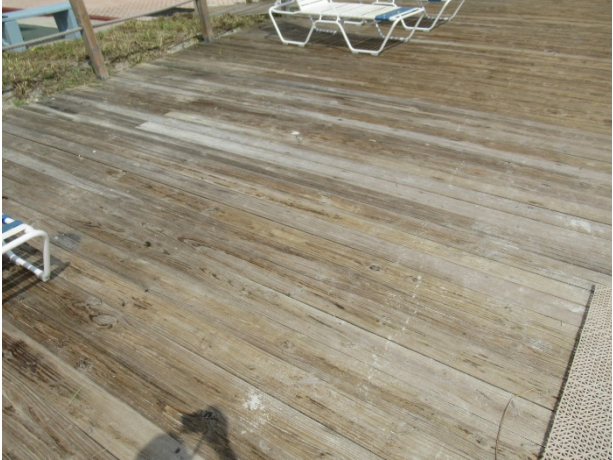
Weathered deck boards
