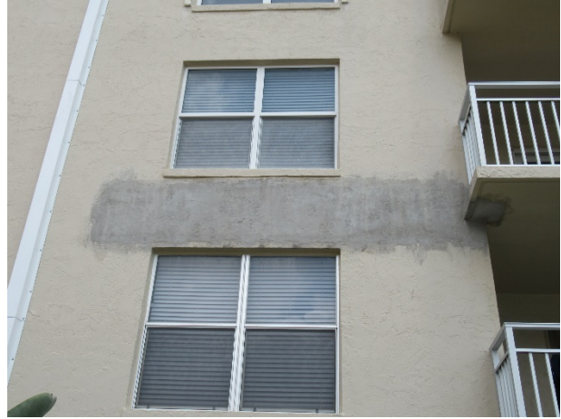
Recent stucco repair
