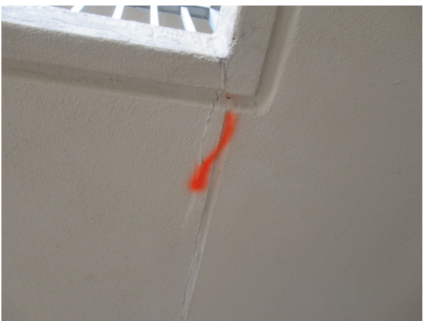
Crack to breezeway underside to be repaired
