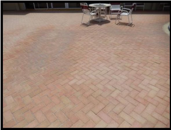
Figure 14 Pool Deck Wear
