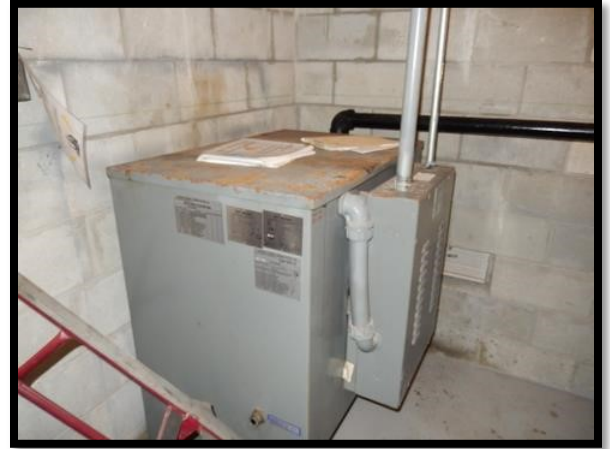
Figure 47 Laundry Tub and Water Heater
