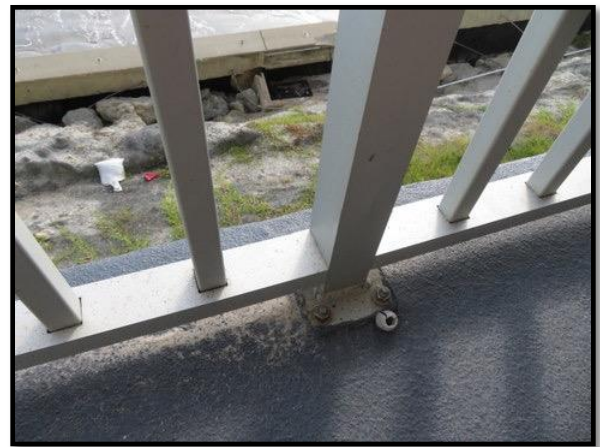
Figure 2 – Balcony Railing Caps Missing
