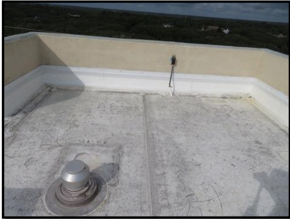
Figure 1 – Rooftop Knee Wall Needs New Paint
