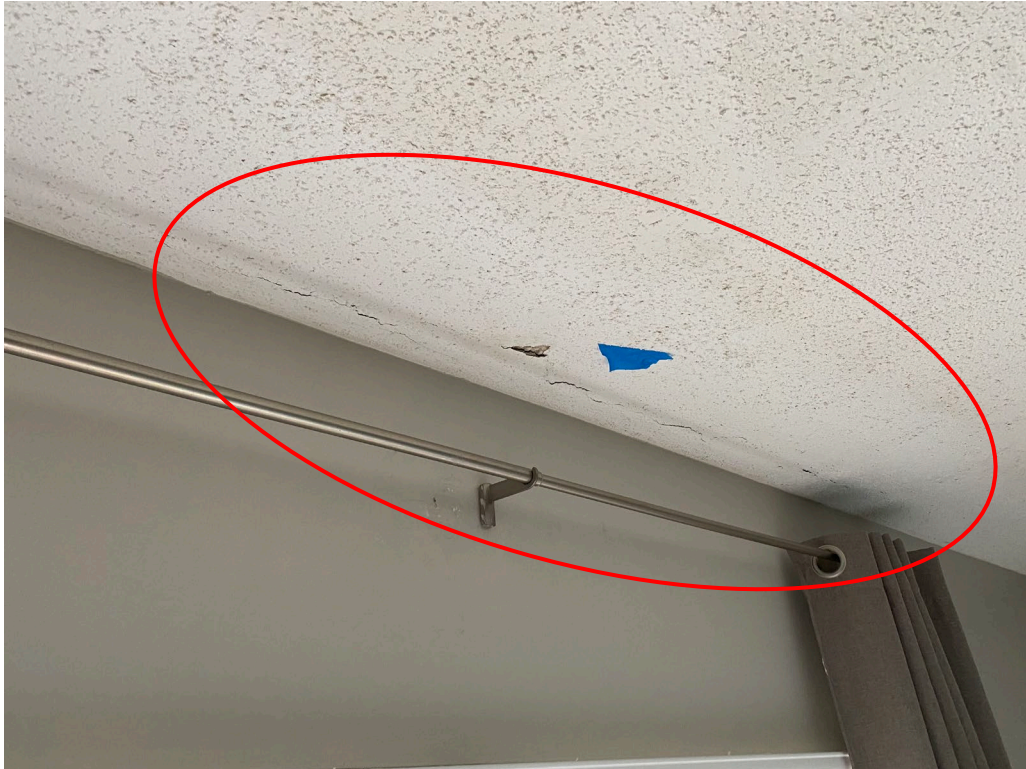
Photograph #1 – Typical interior ceiling concrete spalling damage
